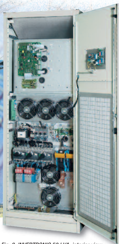
Fig. 3: INVERTRONIC 50 kVA, interior view
